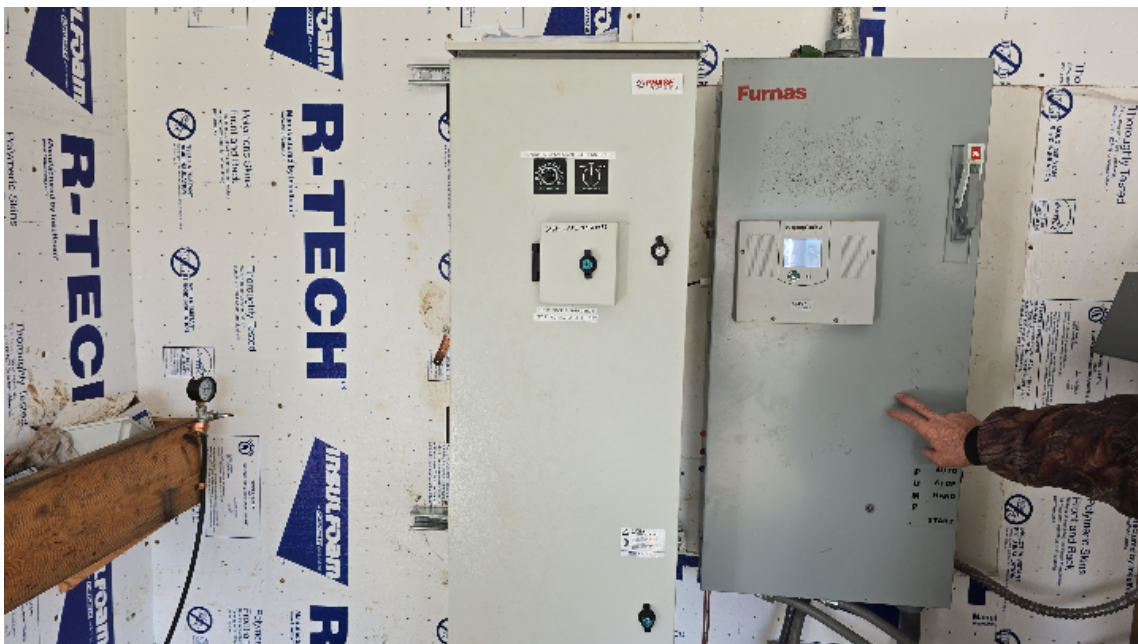
General Site - Station 1, Variable Frequency Drive
