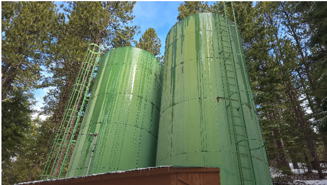
General Site - Station 4, Tanks, 30,000 Gal., Mill Creek
