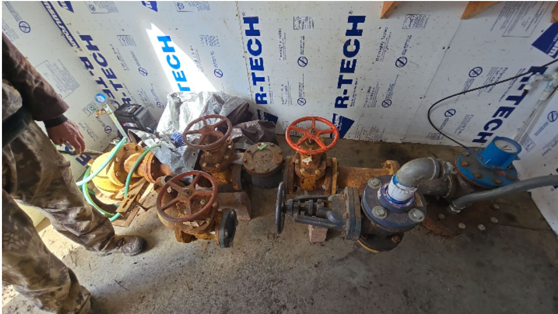
General Site - Station 1, Pumps & Controls
