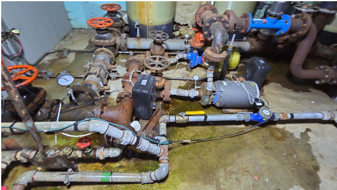
General Site - Station 2, Pumps & Controls
