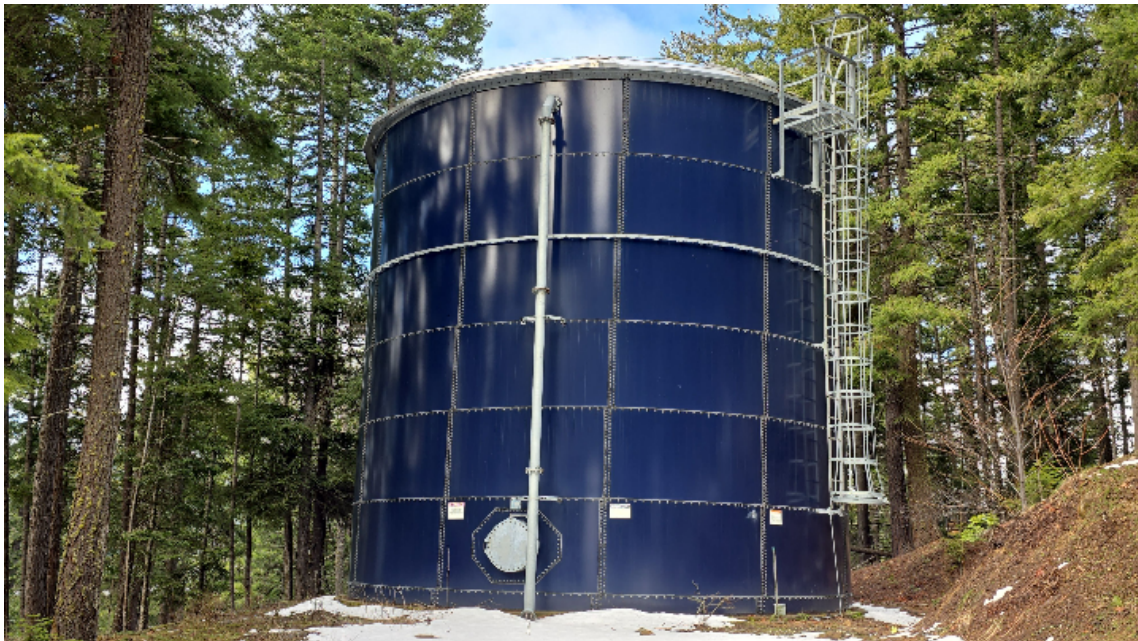
General Site - Station 3, Tank, 40,000 Gal., Highland Drive Reservoir
