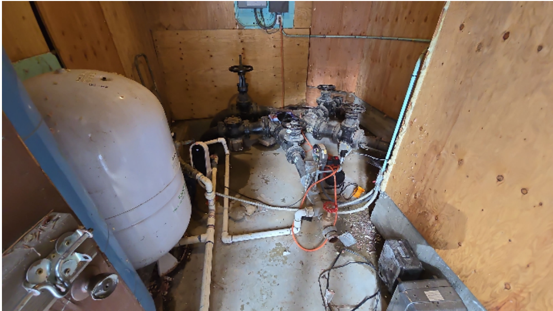
General Site - Station 4, Pumps & Controls, Mill Creek
